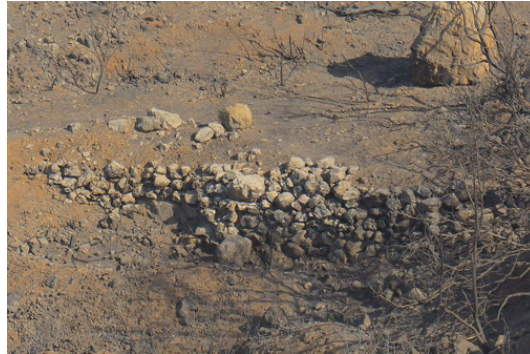
Figure 1, Dry stone wall revealed in the denuded landscape immediately after the fires of 2021.
